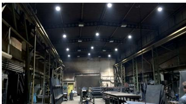
po instalaci HIGH-BAY
